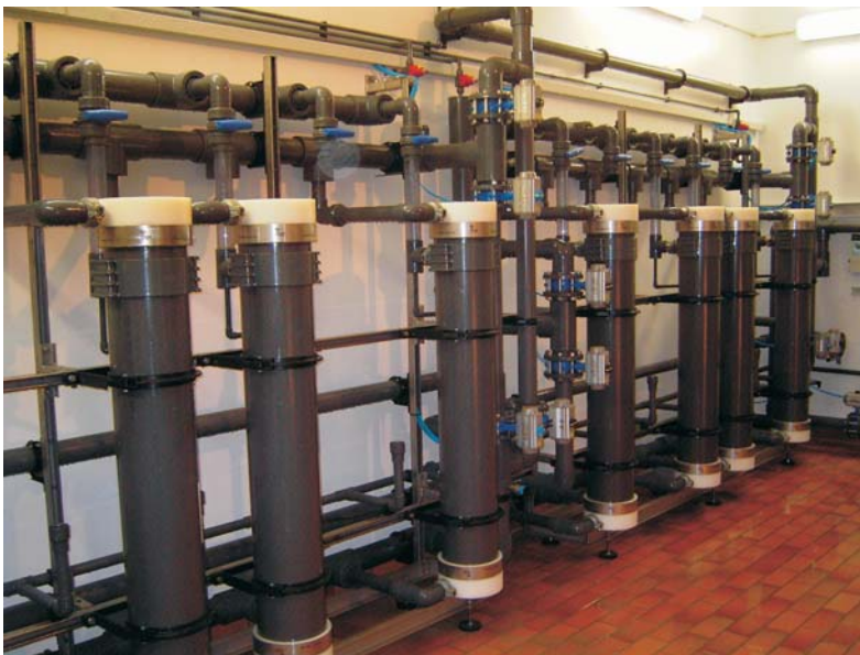
(Spring water preparation: high-level reservoir Michelbach: 30 m 3 /h)
